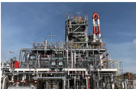
Pilot facility to produce ethylene from renewable ethanol
